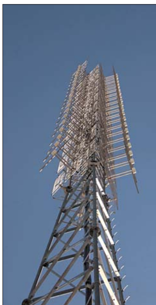
The Shively Panel antenna mounted on the tower.
