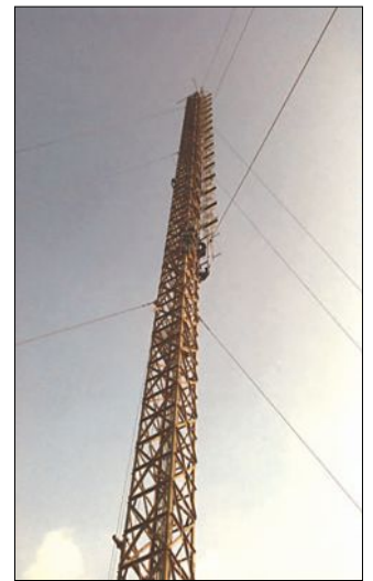
The Antenna on the Tower
